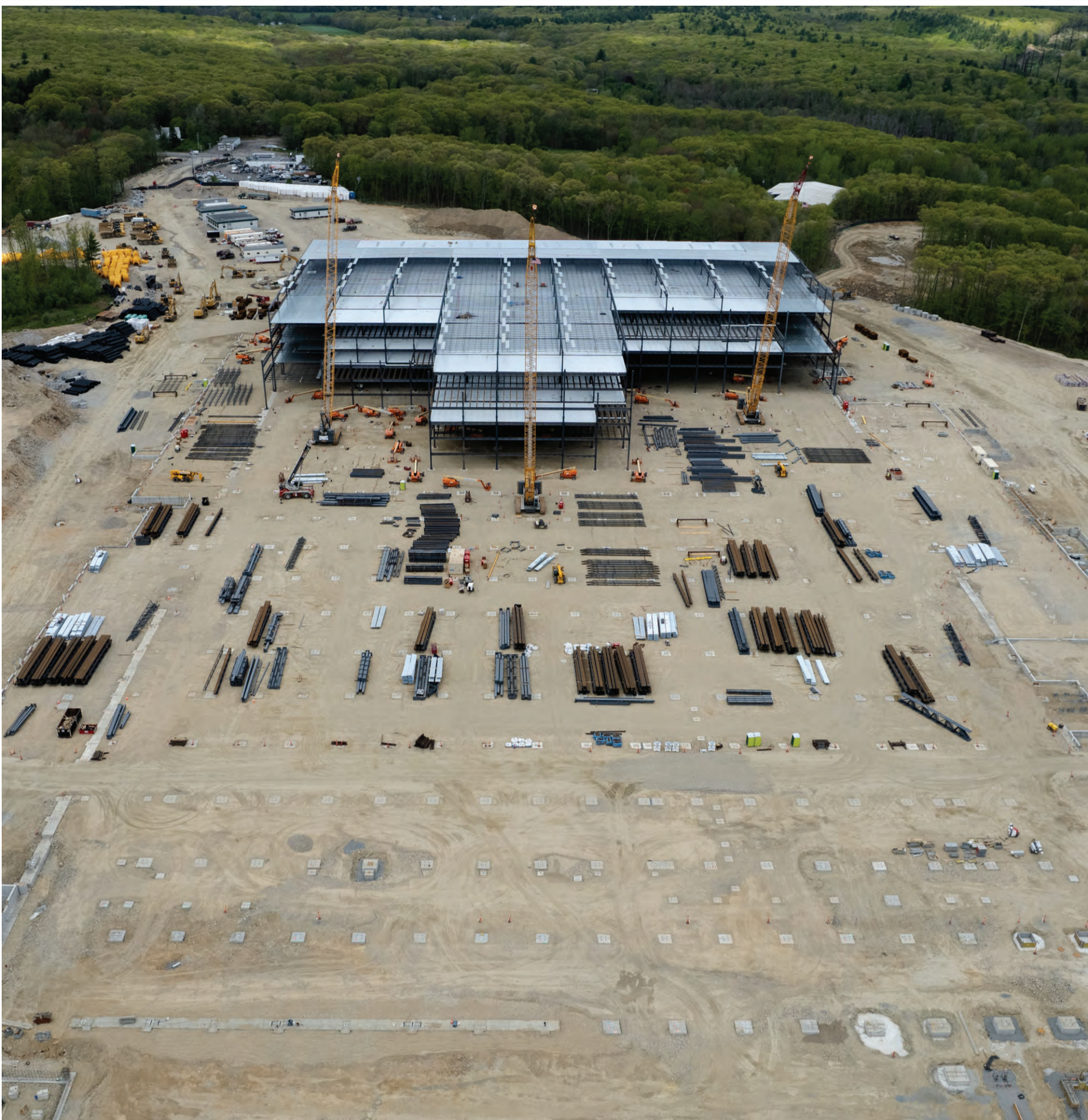
BIRD'S EYE: These images of the Amazon construction site in Johnston were captured by drones piloted by Trevor Bryan, an FAA Licensed and insured drone pilot, the owner and operator of New England Aerial Services, on May 15. For more information on the Warwick-based company, visit their Facebook page at www.facebook.com/newenglandaerialservices . For more aerial photos from the Amazon site, go to www.johnstonsunrise.net . (Photos courtesy New England Aerial Services)
